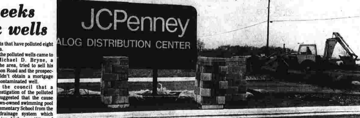
Landscaping under way Construction continues and landscaping is under way at the site of the warehouse which is the major occupant of the Buckland Industrial Park to which townspeople look for new sources of tax revenue and employment. (Herald photo by Pinto)
